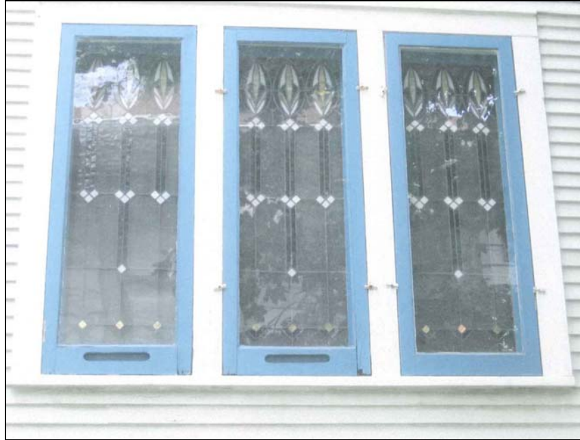
Detail of casement windows in bay on North façade (Photo source: Katharine Keleman, 2006)
