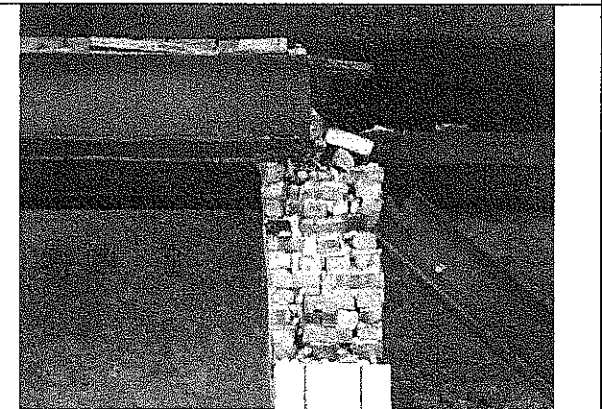
Picture 6 – 2011.08.10 Photo showing terra cotta missing under beam flange resulting in loss of bearing surface for beam
