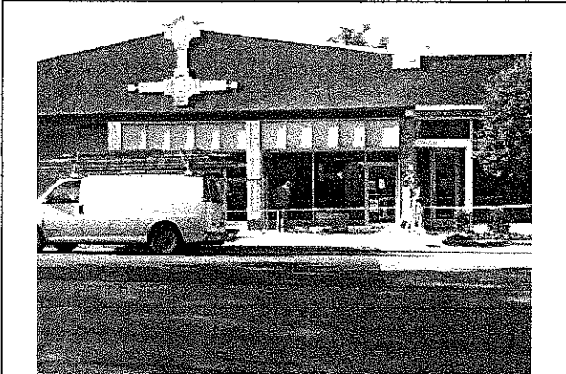
Picture 3 – 2011.07.07 Photo showing un-permitted work underway – removal of terra cotta at pier, terra cotta trim & soldier brick course at lintel. Note there is no electrical junction box at surface of exposed brick near top of pier
