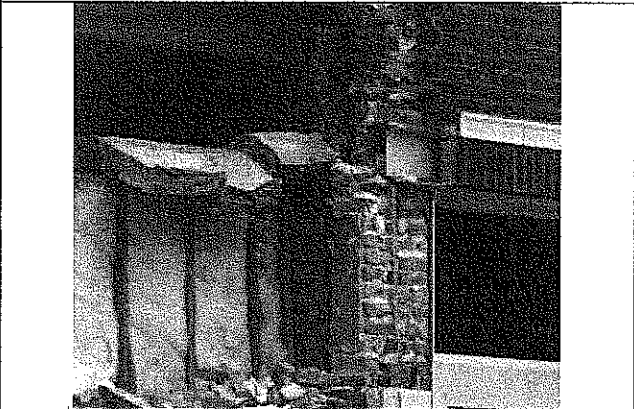
Picture 5 – 2011.08.10 Close-up of top of pier showing unpermitted electrical work after unpermitted terra cotta removal and replacement & loss of bearing for beam due to removal of terra cotta
