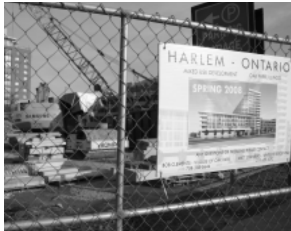
Apartments, townhomes, parking and a Trader Joe's specialty market will soon rise on this site at Harlem Avenue and Ontario Street.
